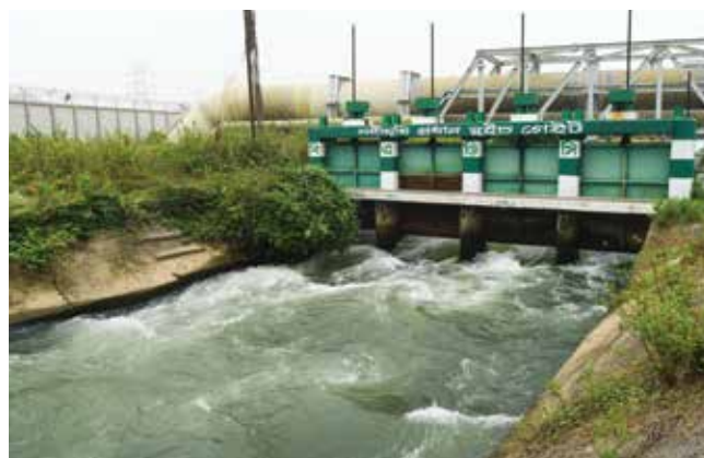
Ashuganj Power Plant Intake Point
