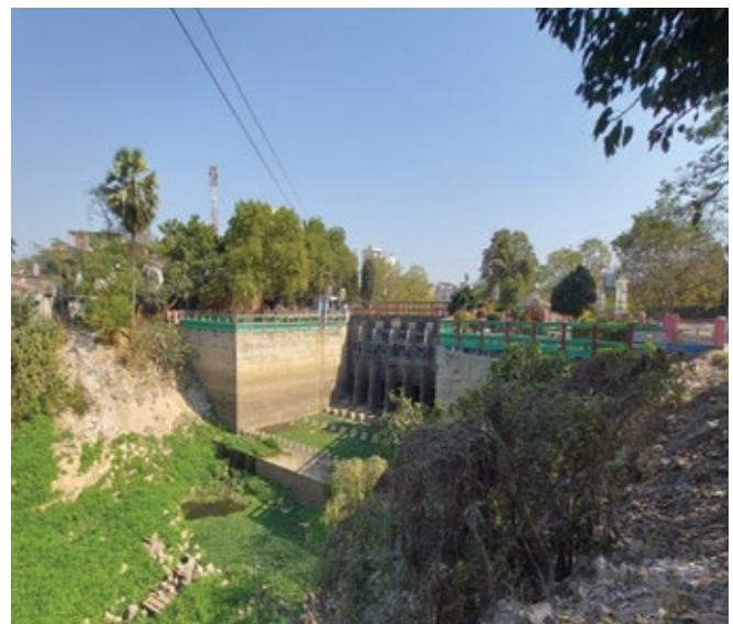
Non-functional Regulator at Robanpur, Chapainawabganj
